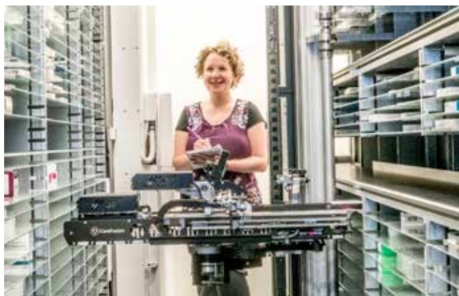
Opposite: Pharmacists Nicole Kirby and Lauren Maxwell. Above: Pharmacist Marissa Izzard with Barwon Health's robotic system for dispensing medications, the first of its kind to be installed in an Australian health service.
